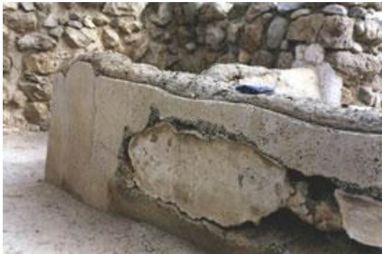
An earlier intervention with white cement causing evident damage on this ancient mud brick and lime
