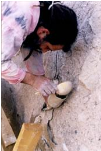
Filling of the voids from all directions with liquid mortar made of NHL - 2 and pieces of light-weight high fired ceramic balls and ancient pottery sherds
