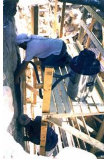
The careful cleaning of the huge void after securing the panel with lime fasteners and gauze with weak solution of acrylic resin
