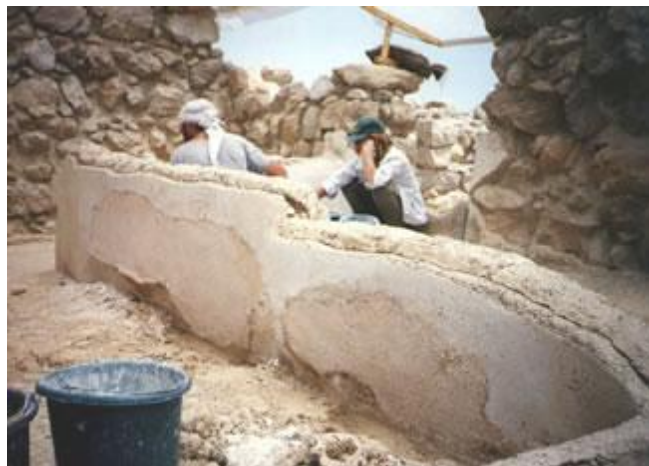
Consolidation of mud bricks and integration to original. The same wall after having removed the cement and replastered with NHL 2
