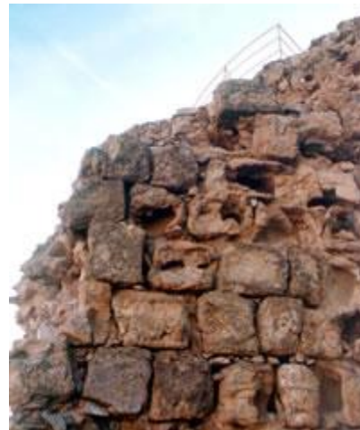
Soft-stone facade deteriorated to point of collapse.
