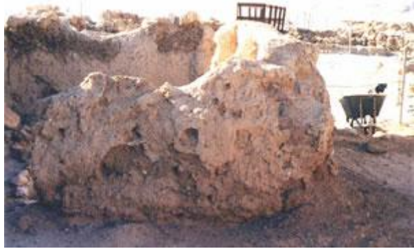
A badly deteriorated mud-brick and mud plastered wall
