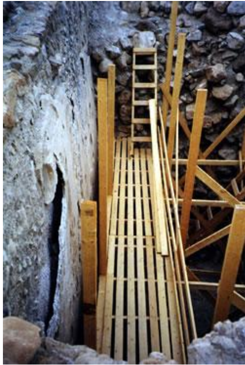
The large panel on the wall of the grand pool detached by uncontrolled flood waters from above.
