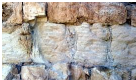
Filling of limestone tiles bedded in an NHL 2 mortar in cavernously decayed soft limestone. The pointing uses NHL 2 mortar with limestone pins.
